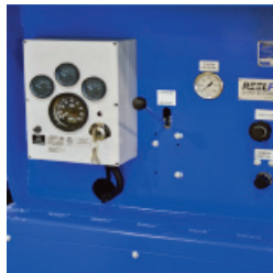
Centralized Control Panel
